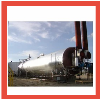
Crude Oil Heater
