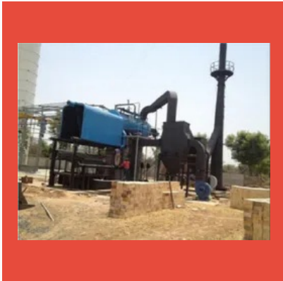
Coal Fired 600 kg/hr Fluidized Bed Combustion (FBC) Boiler
