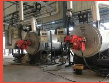
Thermic Fluid Heater
