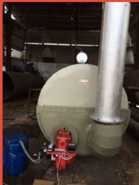
Indirect Water Bath Heater
