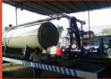
Diesel Fired Indirect Heating
